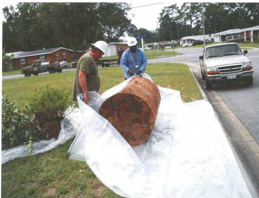
Picture 2: UST 1252Dove.
